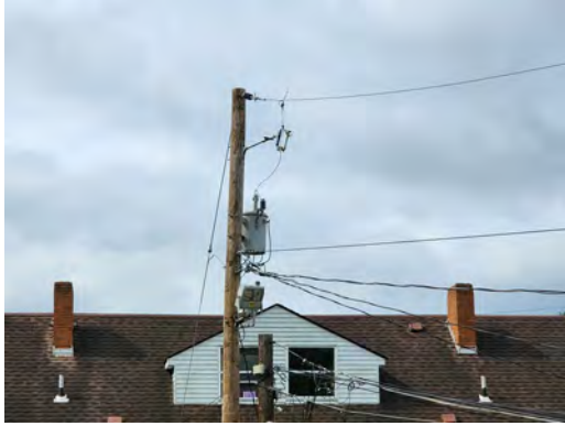
PHOTO #31 POLE-MOUNTED TRANSFORMER
