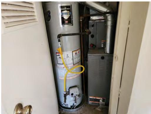
PHOTO #29 TYPICAL RESIDENT UNIT FURNACE AND WATER HEATER
