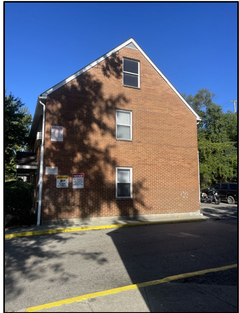
16. Representative view of side of existing apartment building within the project site, looking west.
