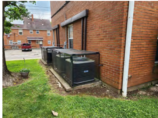
PHOTO #28 AIR CONDITIONING UNITS
