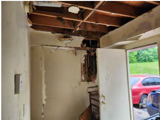
PHOTO #27 WATER DAMAGE
