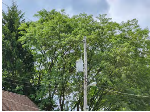
PHOTO #32 POLE-MOUNTED TRANSFORMER
