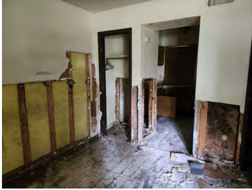
PHOTO #25 RESIDENTIAL UNIT WITH SUBSTANTIAL WATER DAMAGE
