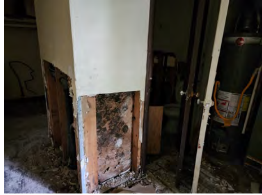
PHOTO #26 MOISTURE INTRUSION AND SUSPECT MOLD
