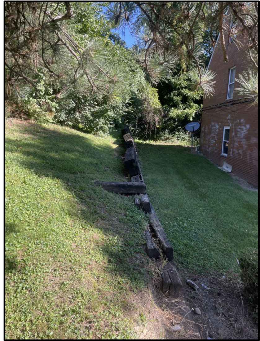
10. View of existing dilapidated retaining wall to be replaced within the project site, looking north.
