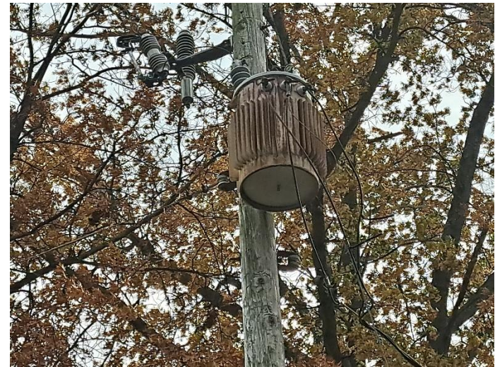
Photo 8: Pole mounted transformer located on the east portion of the Subject Property.
