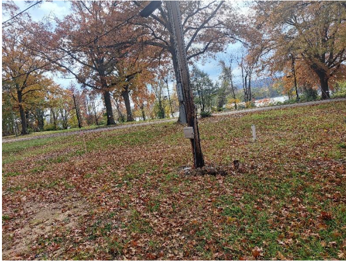
Photo 5: Typical electrical hook up located throughout the Subject Property.
