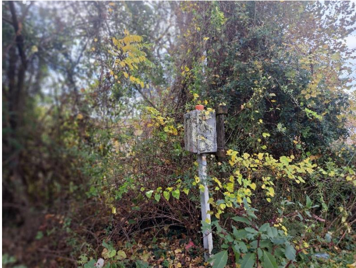
Photo 7: An apparent lift station located near the southwest corner of the Subject Property.
